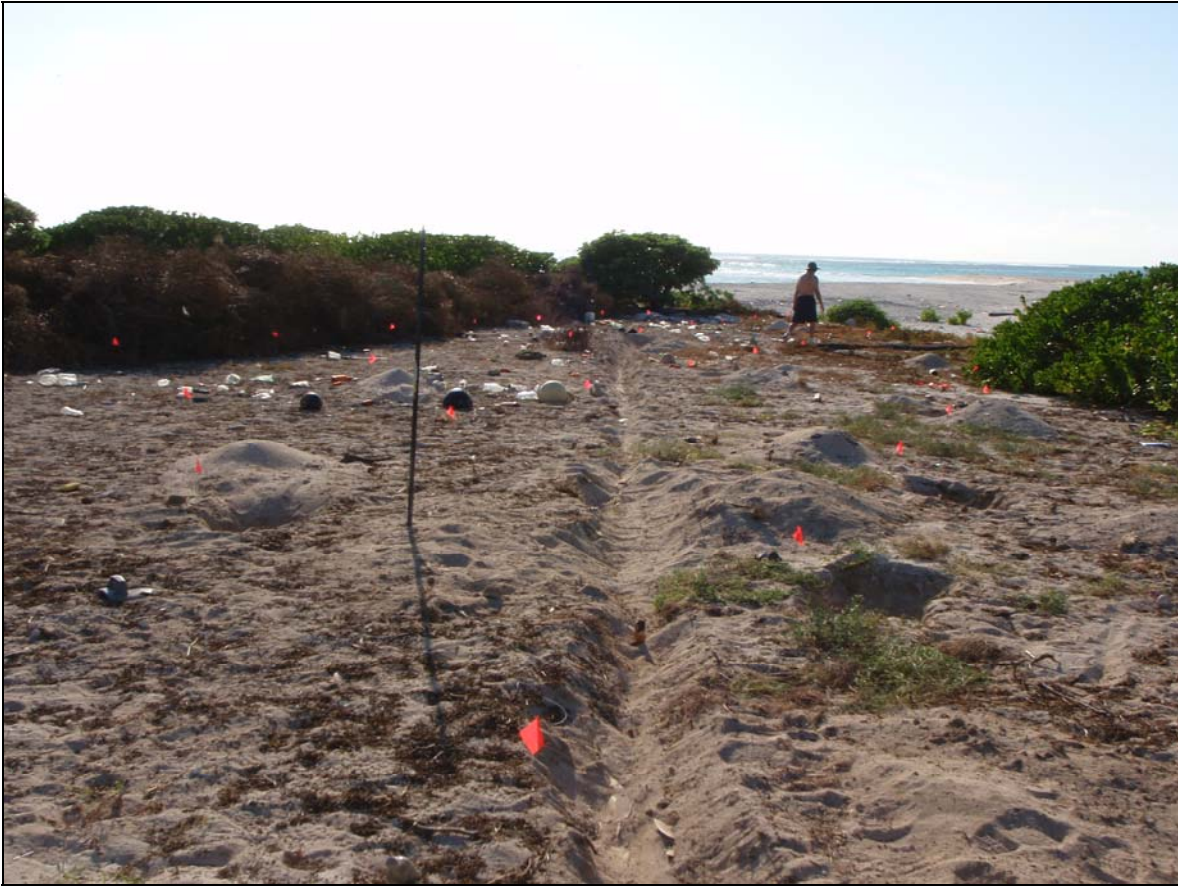
Pipeline located within SMD.
