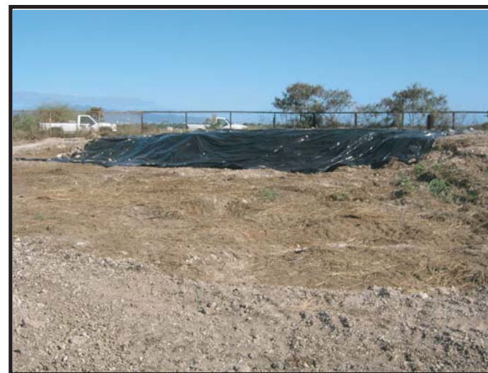
Photo 12: View of polyethylene sheeting placed over SA3 after sample collection to minimize storm water infiltration
